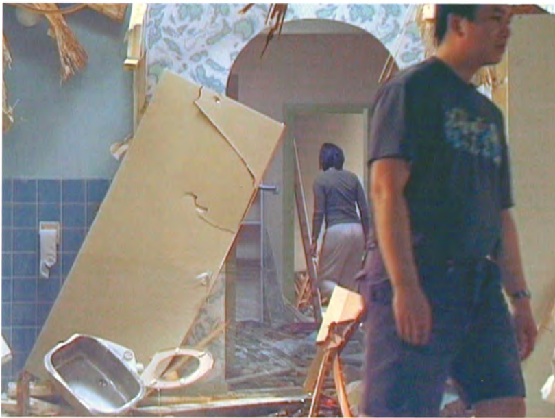
Softer Catwalk in Collapsing Rooms, 1999
